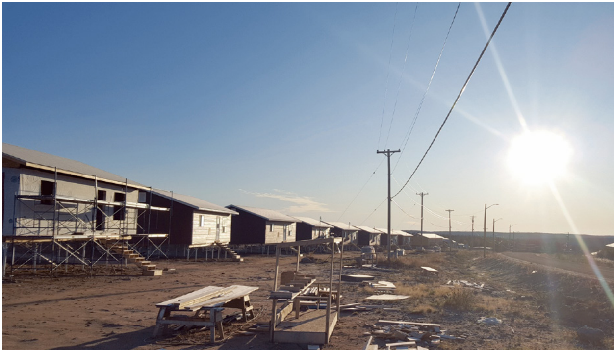
Homes under construction in October 2019 on Marcel Colomb First Nation (Black Sturgeon), 320 kilometres northwest of Thompson. The Stantec Conservation and Efficiency study recommends increasing the available funding and access to funding for Northern communities for water distribution system operations and maintenance. Photo: Ph Gorzen/Wikimedia Commons
