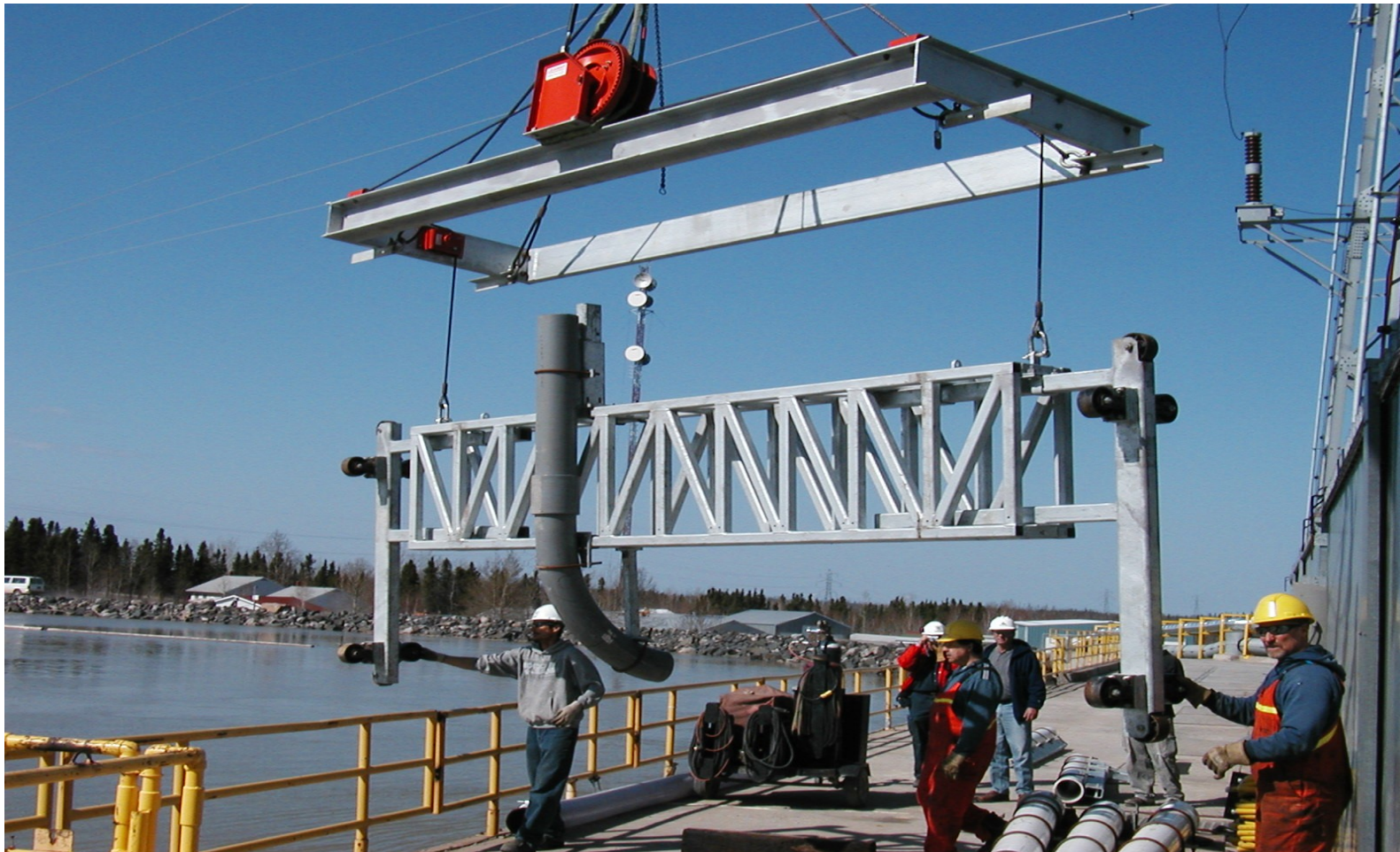
Figure 2-10. Steel support frame and lower section of the 20 cm diameter PVC release pipe used to release fish into Unit 2 intake at the Kelsey GS (2006 photo).
