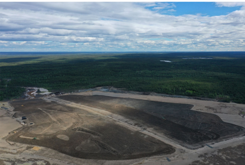
Tailings Management Area 3 (TMA 3) – The clay is in place and work is underway to dry and compact to create the protective Clay Cap.
