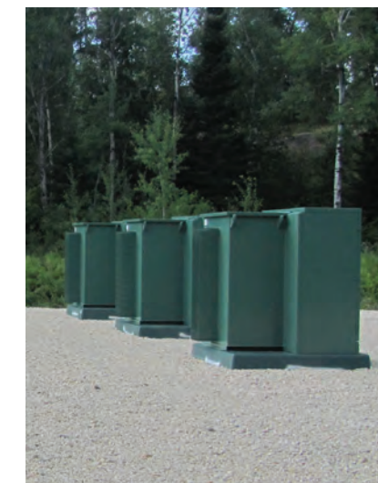
Regulators at the Pointe du Bois Distribution Supply Centre.
