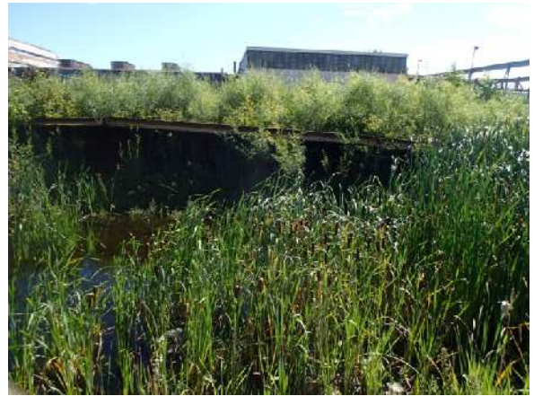
Figure 02 – Facing east at leaning retaining wall from west bank
