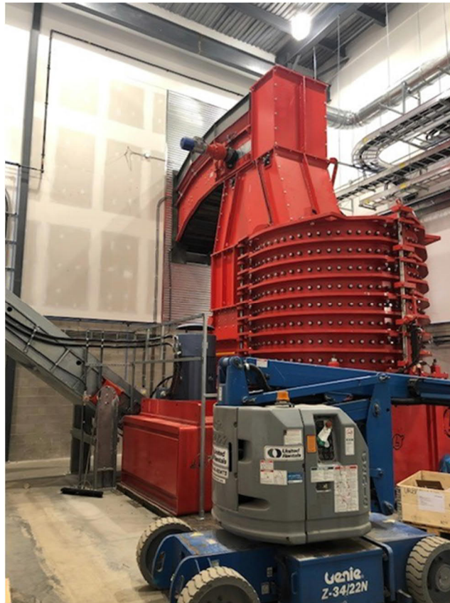
Photograph 2: Bano Vertical Mill
