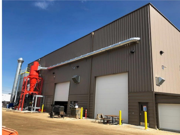
Photograph 4: Cyclone and Baghouse
