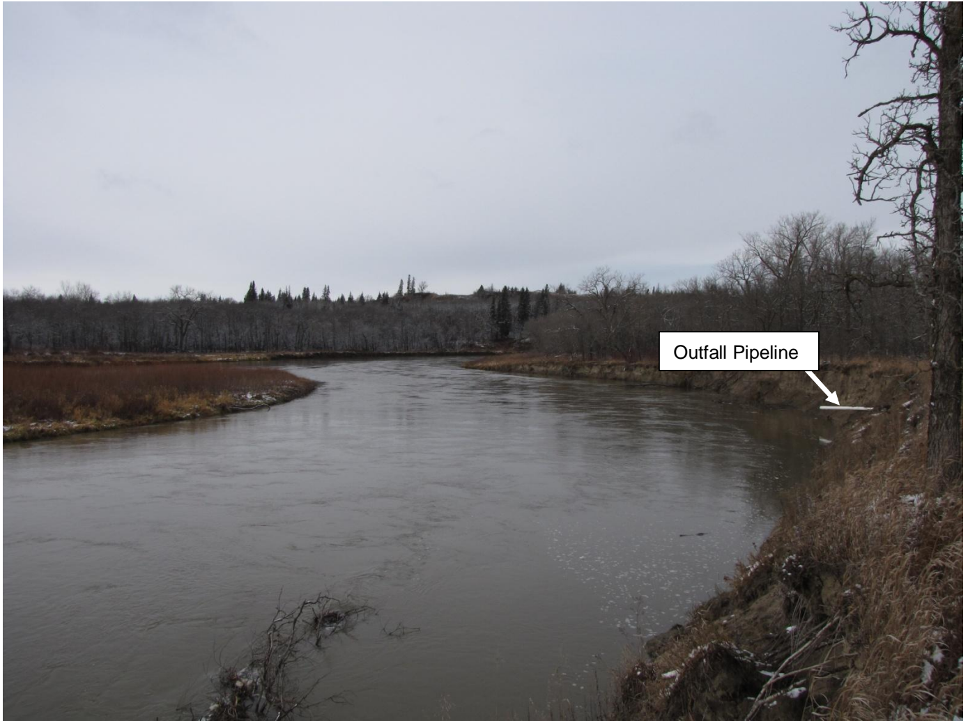
Photograph 4. Facing north showing the existing lagoon discharge pipe on the right hand side of the photograph ↑
