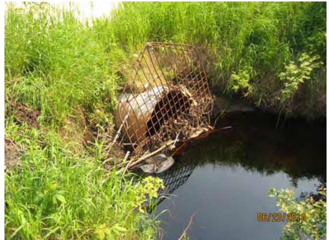
Photo 6. Grate on upstream side of culvert at the water crossing under Grindstone Rd.; effectively blocking fish passage of large bodied fish.
