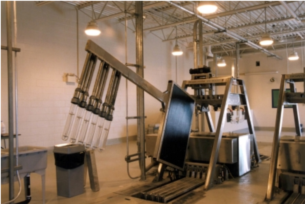
UV Disinfection Lamp Systems at SEWPCC Figure 4-2
