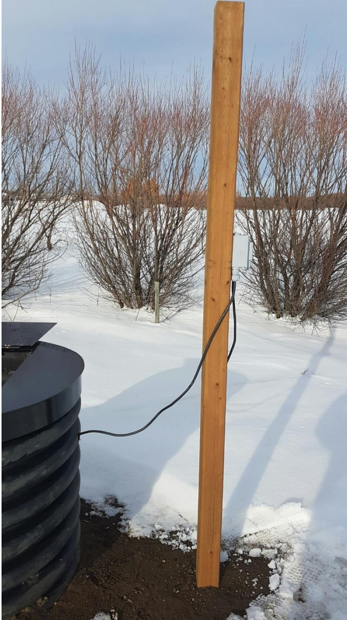
Photo #5 Sump electrical hookup (January 31, 2017).
