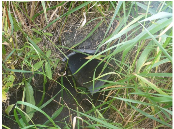
Photograph 8 ↑ Existing effluent discharge pipe located along the western berm of the existing secondary lagoon cell.
