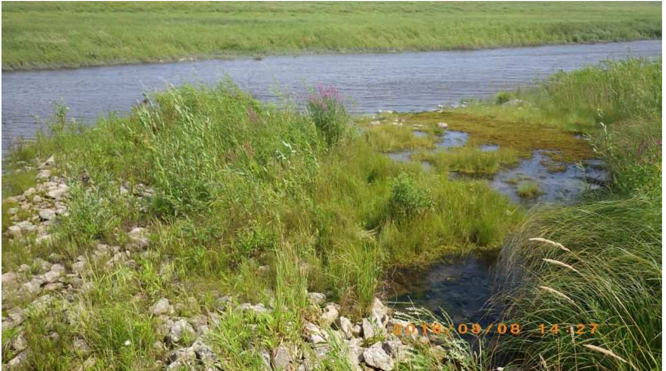
Photo 2: Water finding alternate flow path to LFC at 8B2.
