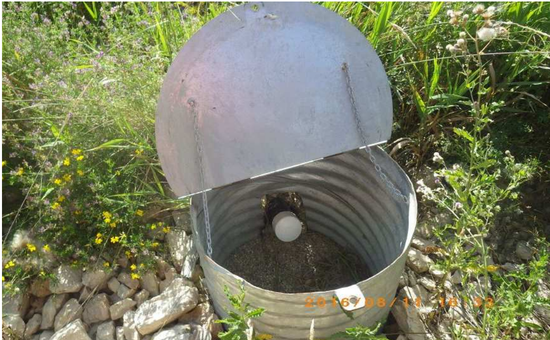
Photo 1: High level sampling pipe and protective CMP casing.
