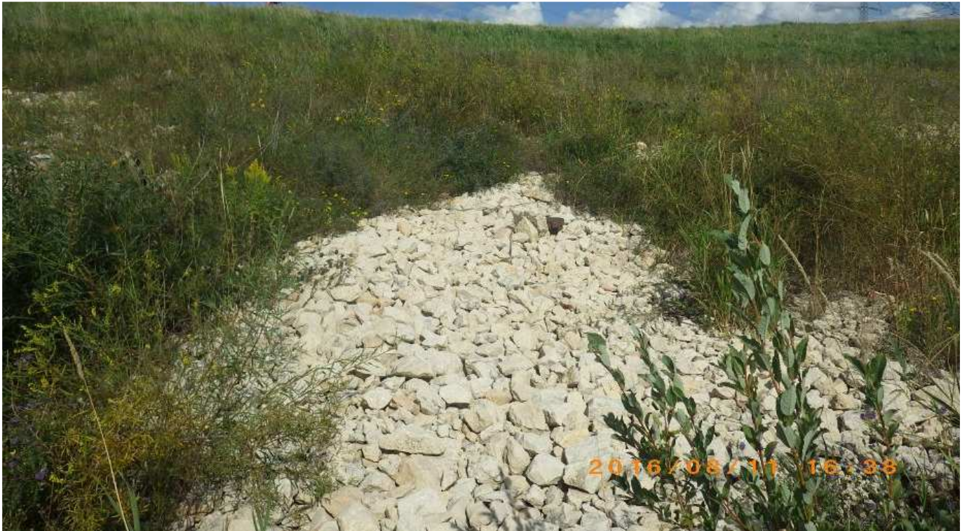
Photo 2: Water flowing through 11A2 filter and finding alternate flow paths to LFC.
