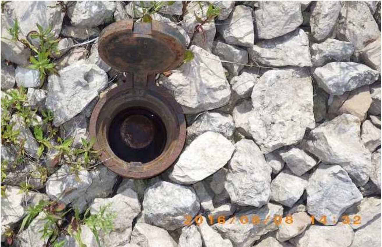
Photo 2: Low level sampling pipe and protective steel casing at 8C1.
