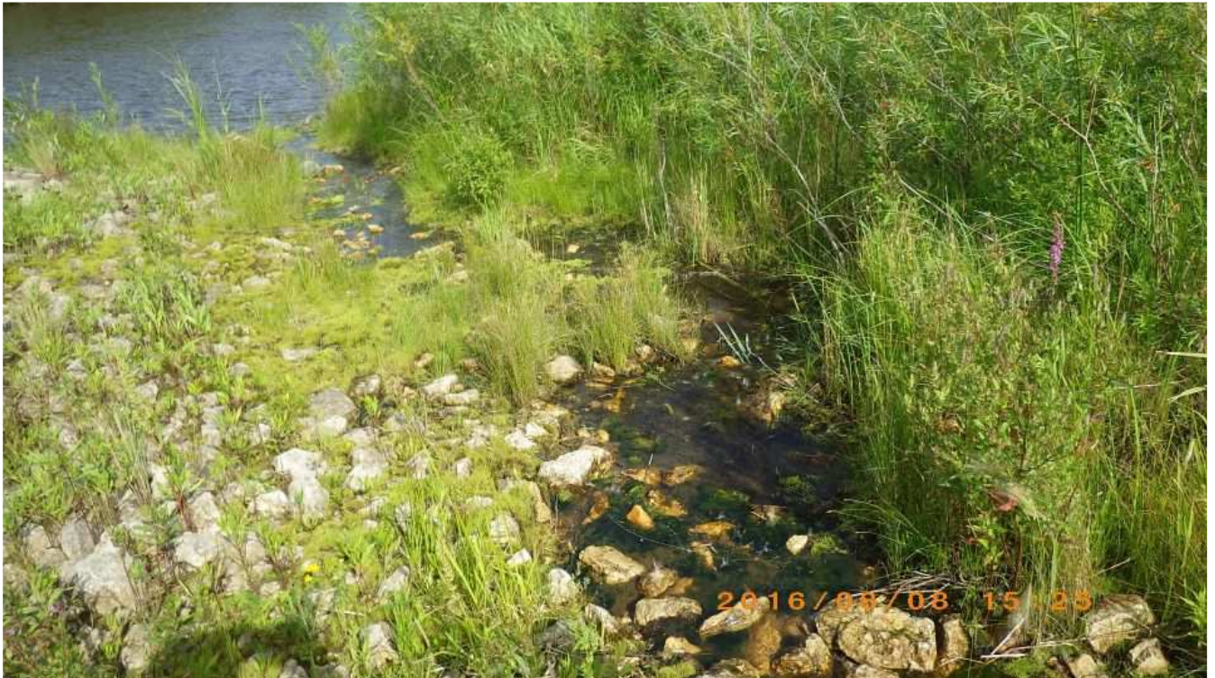
Photo 2: Water flowing through 10A1 filter and finding alternate flow paths to LFC.
