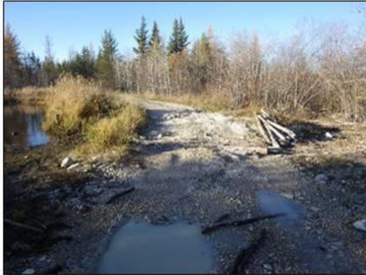
Figure C-7. Access road at Crossing 2. Road was washed out prior to clearing and grubbing of culvert.
