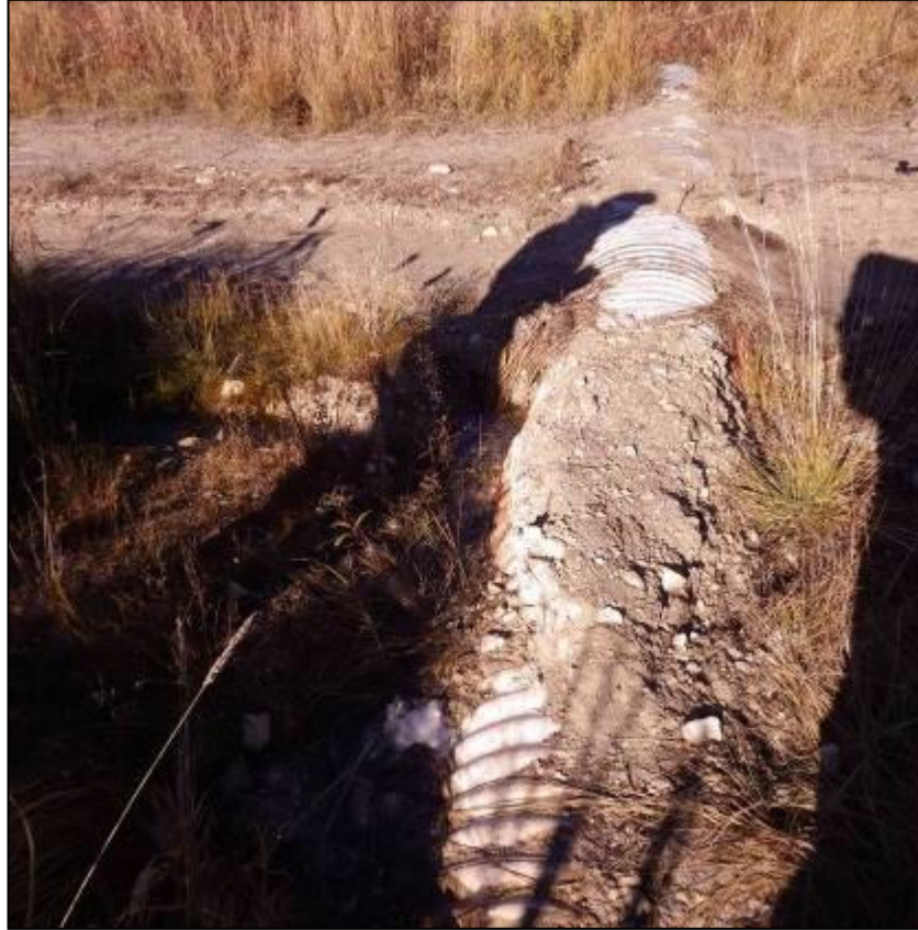
Figure 6. One of three culverts at Crossing 3, exposed across road and completely blocked at upstream end.
