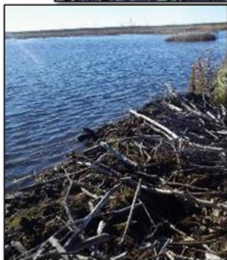
Figure B-4. Upstream (left) and downstream (right) views of Culvert 3B. The upstream side was completely buried in woody debris and the downstream side was somewhat damaged.
