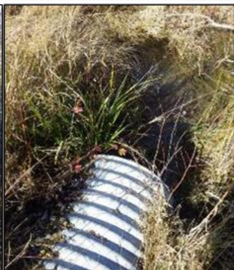
Figure B-5. Upstream (left) and downstream (right) views of Culvert 3C. The upstream side was blocked by debris and vegetation; blockage resulted in water flowing across the road.
