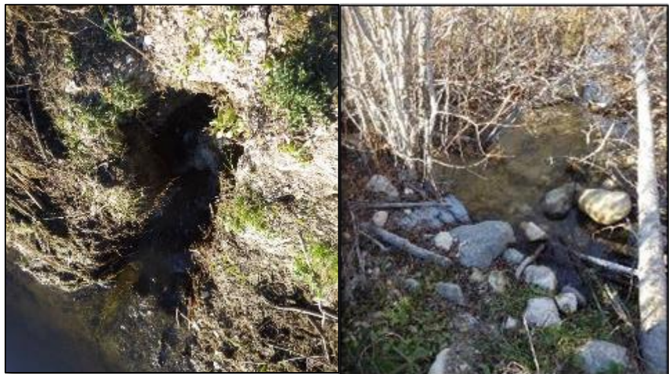
Figure B-2. Upstream (left) and downstream (right) views of Culvert 2 shortly after clearing.
