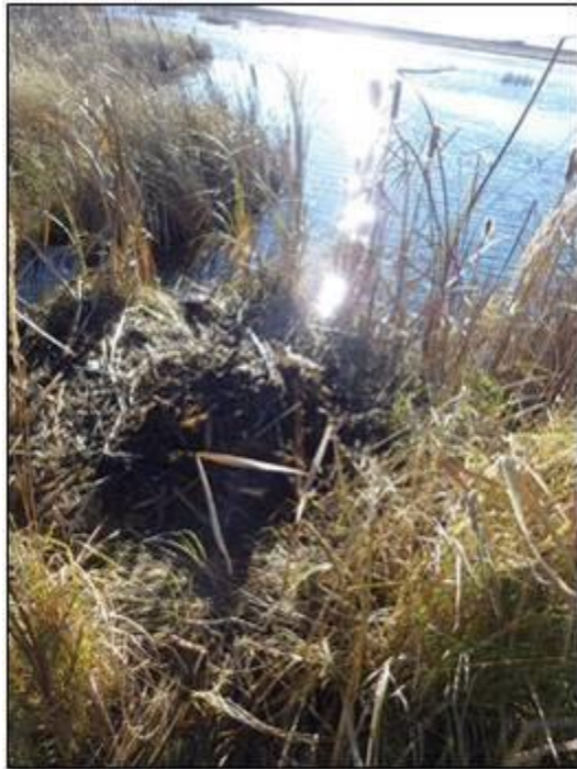
Figure C-16. Plugged culvert at Crossing 3.
