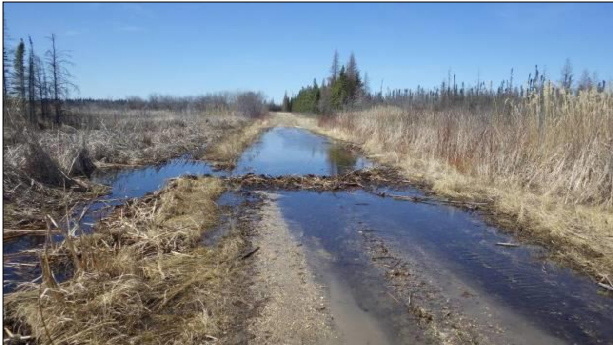
Figure 7. Washout of existing access road north of Crossing 2 in spring, 2016. Beaver activity had increased between fall and spring field seasons, with the beginnings of beaver dam construction across the existing access road.
