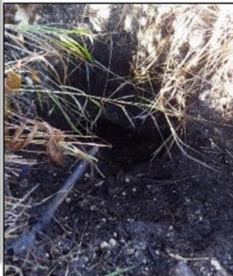
Figure B-3. Upstream (left) and downstream (right) views of Culvert 3A. The culvert was buried deep in the ground.
