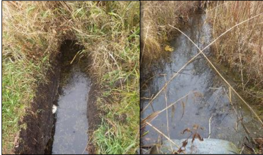
Figure B-1. Upstream (left) and downstream (right) views of Culvert 1 shortly after clearing.
