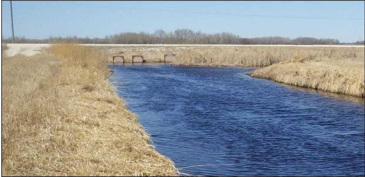
Figure 45. Facing upstream; Closed culverts at the downstream road crossing. The bypass drain enters from the right (east).
