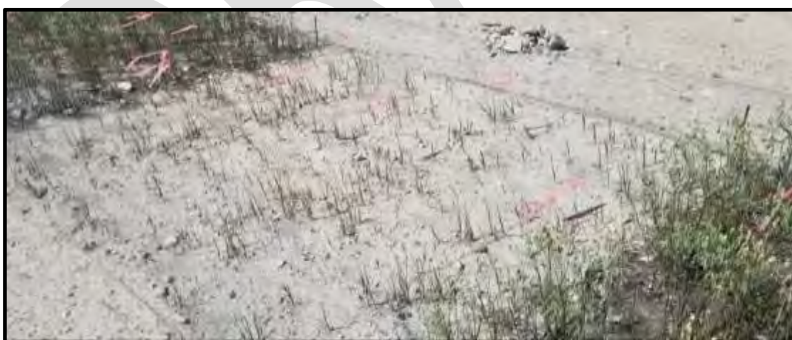
Photo Array 4: Site Inspection – August 8 th , 2019 – Showing summer plant growth – 0.15 m organics depth (top), 0.075 m organics depth (middle), 0 m organics applied (bottom).
