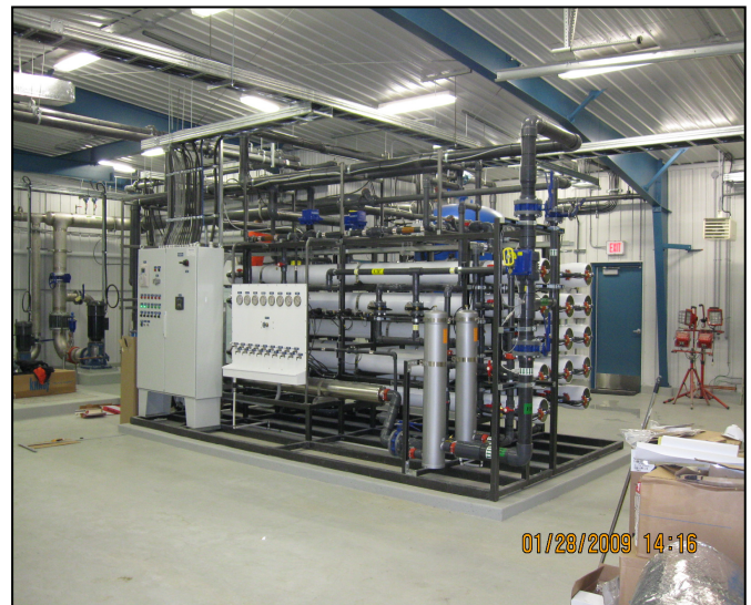
Melita Water Treatment Plant
