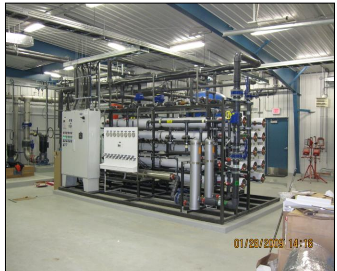
Melita Water Treatment Plant
