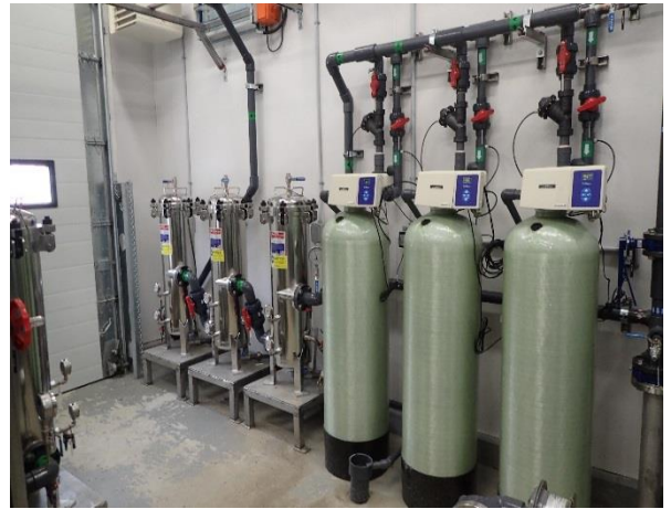
Wekusko Falls Water Treatment Plant
