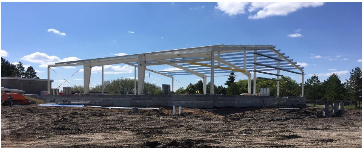
Russell-Binscarth Regional Water Treatment Plant $13.0M
