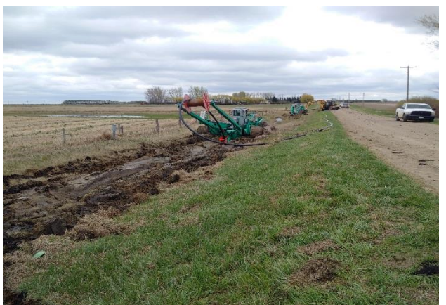
RM of Whitehead Rural Water Pipelines
