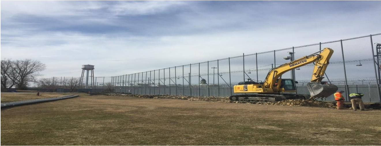
Stony Mountain Institute – Cartier Regional Water Supply
