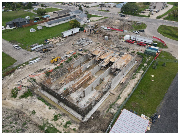
TOWN OF BEAUSEJOUR WATER TREATMENT PLANT
