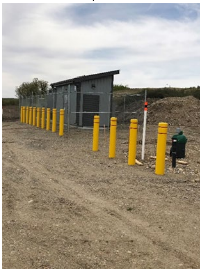
Town of Virden – Well & Pumphouse
