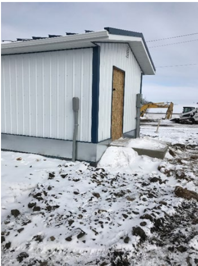
RM of Minto Odanah – Booster Station
