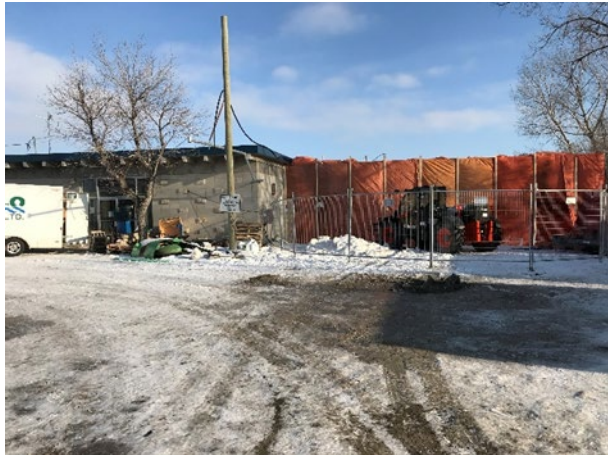
RM of Pipestone – Water Treatment Plant & Reservoir
