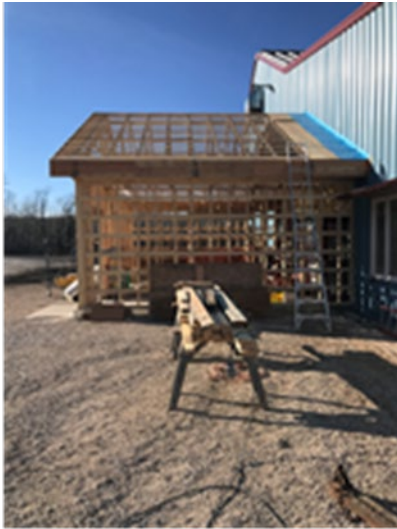
City of Dauphin – UV Upgrades
