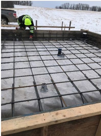
RM of Minto Odanah – Booster Station
