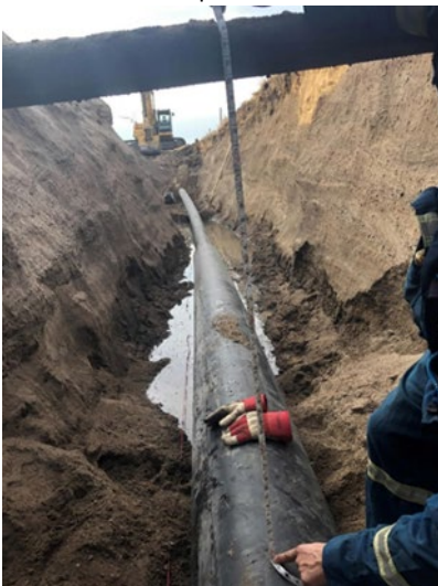
Town of Virden _ Well Mech & Raw Water
