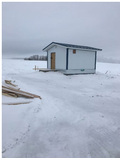
RM of Minto Odanah – Booster Station
