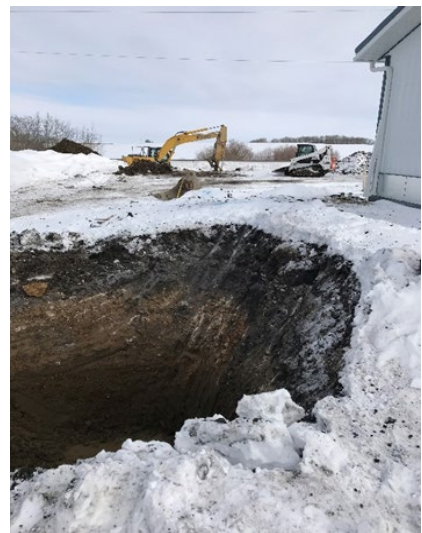
RM of Minto Odanah – Booster Station
