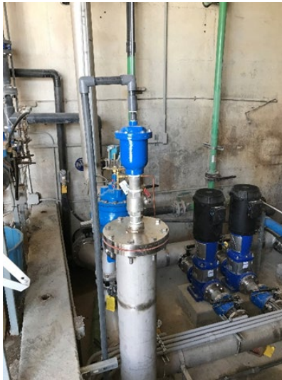
RM of Pipestone – Water Treatment Plant & Reservoir
