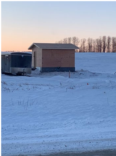
RM of Minto Odanah – Booster Station
