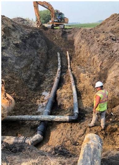
Pembina Valley Co-op Water Supply Pipeline Roland to Winkler
