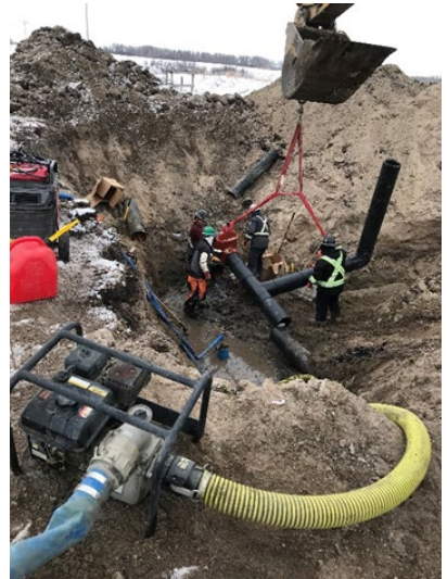
RM of Wallace Woodworth – Raw Supply Flushouts
