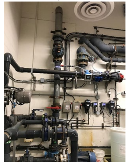
Town of Virden – Water Treatment Plant Piping
