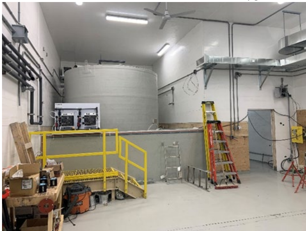
Town of The Pas – Blower Building Chem System
