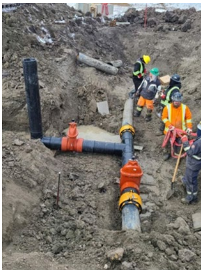
RM of Wallace Woodworth – Raw Supply Flushouts
