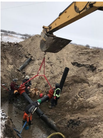
RM of Wallace Woodworth – Raw Supply Flushouts
