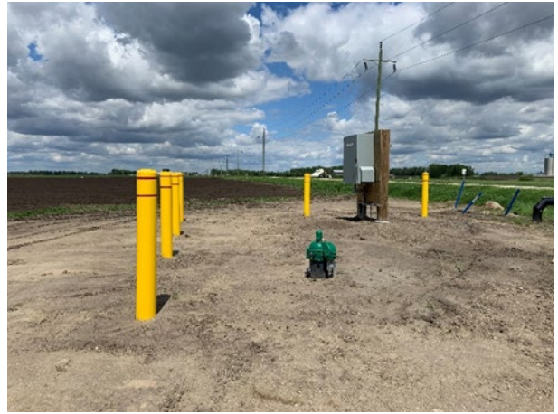
Pembina Valley Co-op – Pitless Booster Station
