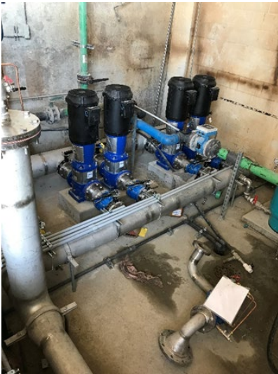
RM of Pipestone – Water Treatment Plant & Reservoir
