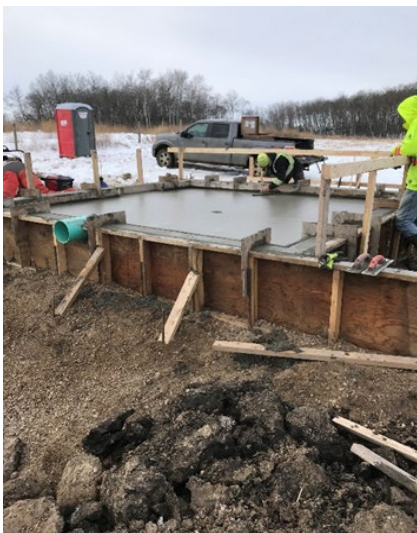
RM of Minto Odanah – Booster Station
