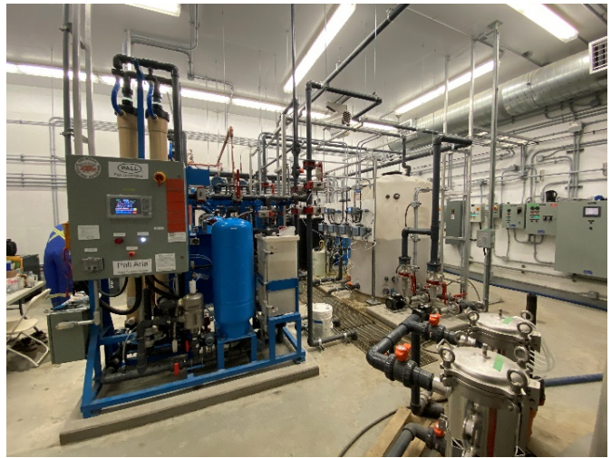
INR Sherridon Water Treatment Plant
