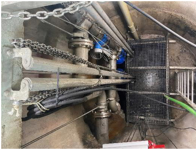
City of Winkler Wet Well
