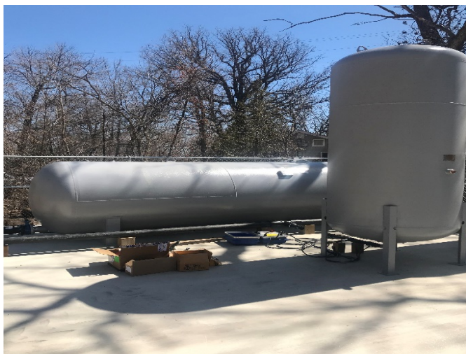
Grand Beach Water Treatment Plant
