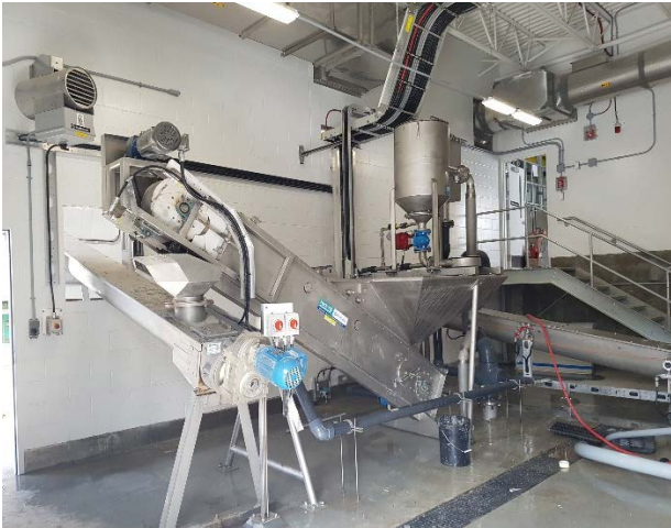
City of Thompson De-Watering Equipment
