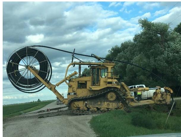
Westlake-Gladstone Rural Pipeline
