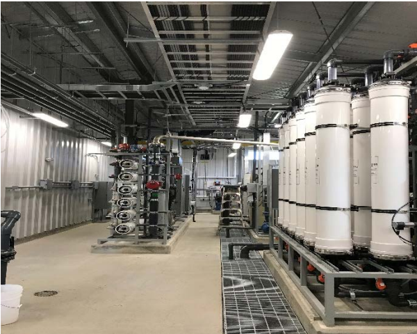
RM of Alexander – Great Falls Water Plant
