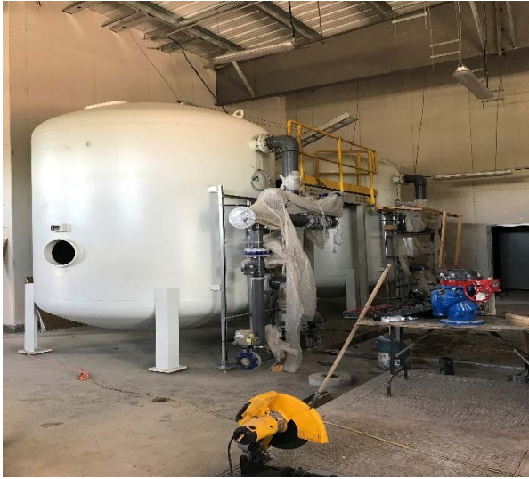
RM of Tache – Landmark Biological Filtration
