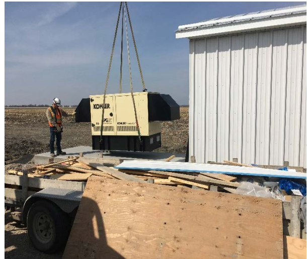
Town of Niverville – Water Supply - Generator
