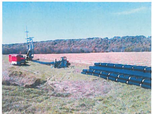
Pilot Mound Water Supply Pipeline
