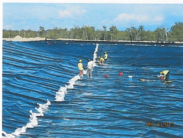
Lawrence Wastewater Lagoon
