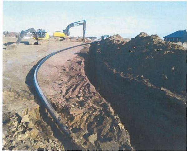
Boissevain Raw Water Pipeline
