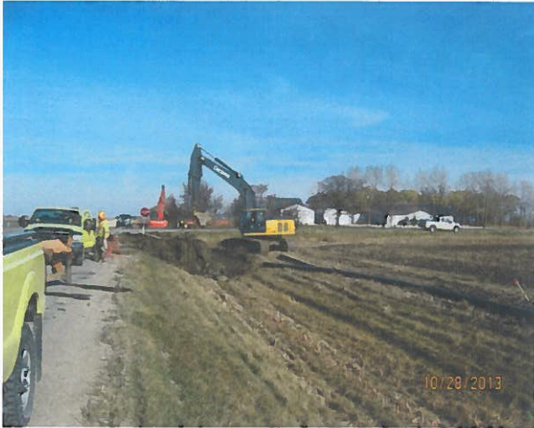
Morris Low Pressure Sewer System
