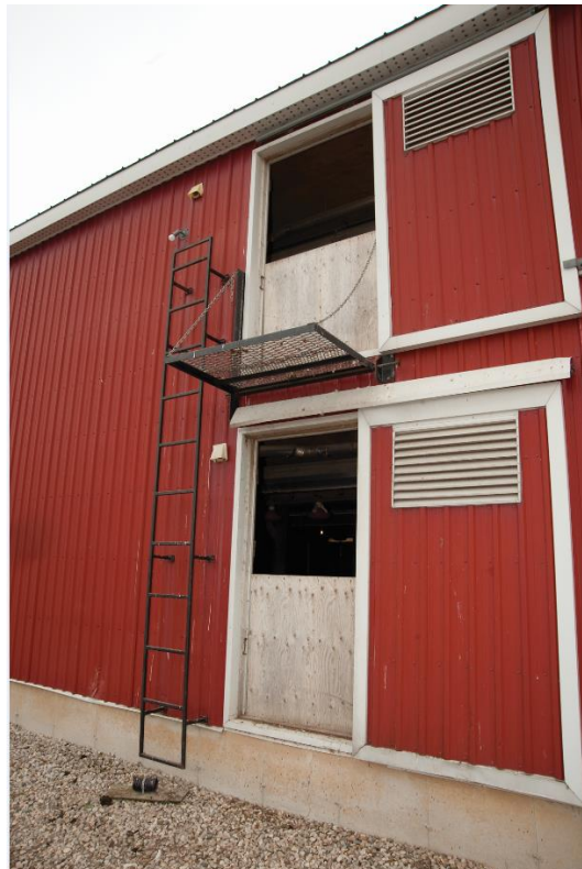
Figure 2.7.2. An example of a fire exit ladder located beside exit doors on a two storey broiler barn. 9
