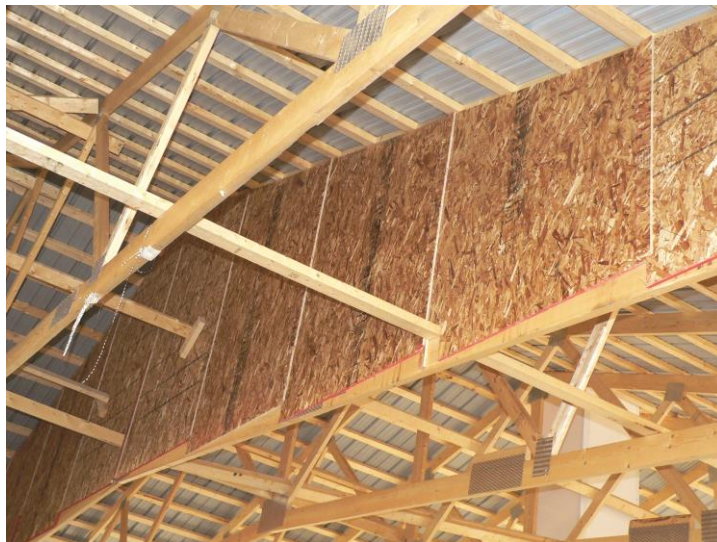
Figure 2.3.2. Example of an attic fire stop under construction in a new calf barn. 6
