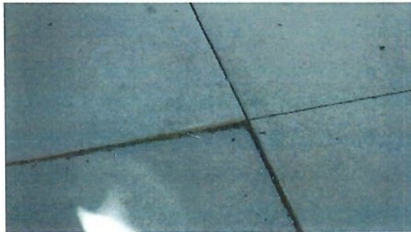
Fig. 7: Example of uneven sidewalk.
