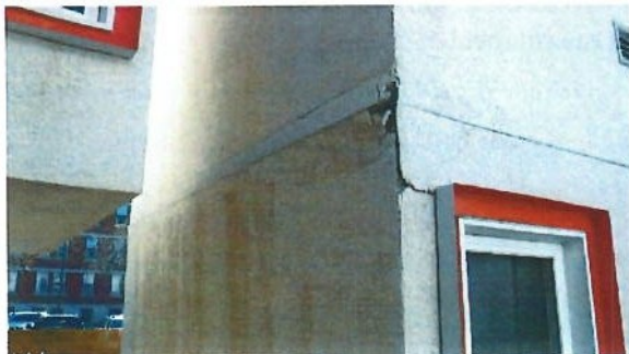
Fig. 3: Damaged wall and stucco due to jacking.
