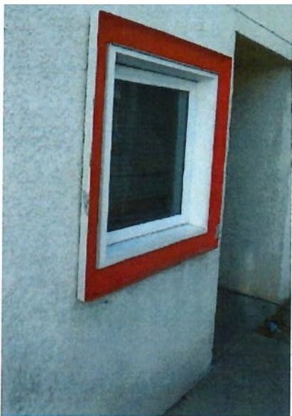
Fig. 14: Another example of peeling trim.
