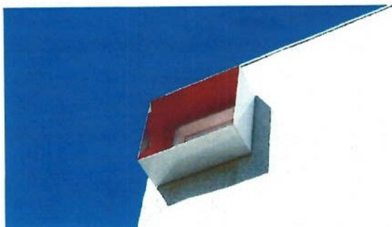
Fig. 13: Peeling window trims.
