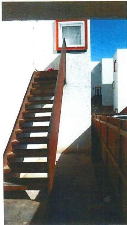
Fig. 11: Example of corroding stairs.
