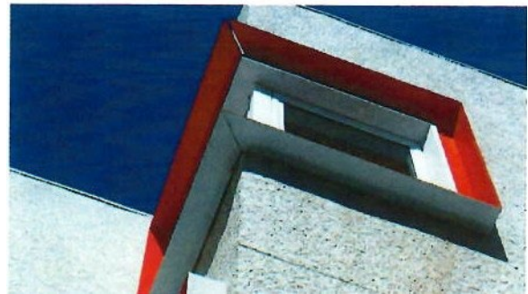
Fig. 15: Split corner in window trim.
