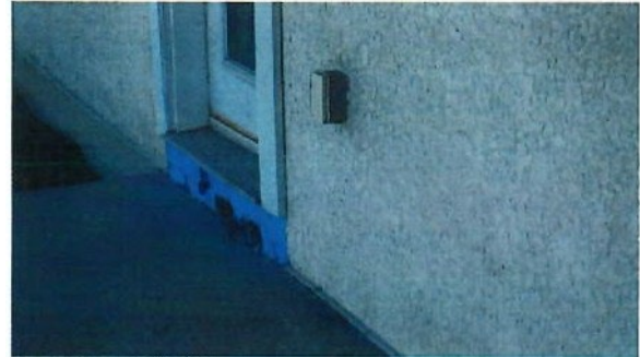
Fig. 9: Example of missing stucco below door.
