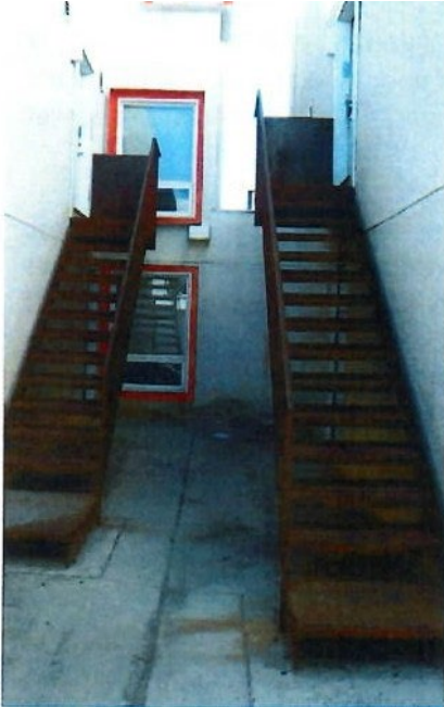
Fig. 18: A typical secluded entrance way where a security assessment may prove beneficial.
