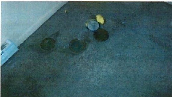
Fig. 6: Floor drain raised out of floor.
