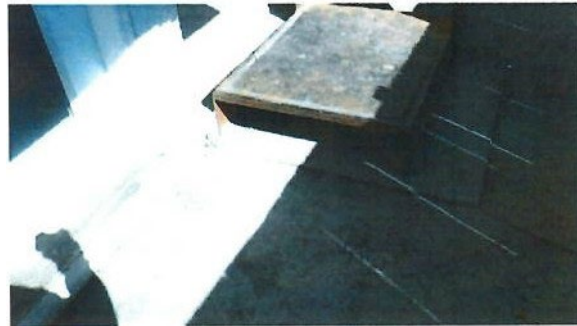
Fig. 8: Multiple elevations to walk through: concrete pad to left of metal platform, metal platform, lower concrete slab, uneven/unmatched sidewalk.
