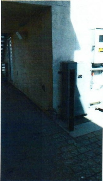
Fig. 10: Example of damaged stucco. Wall patch as well as corner bottom.
