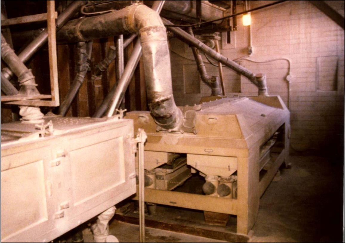
View of a flour purifier in the B.P. Kent Flour Mill (HRB photo, 1991)
